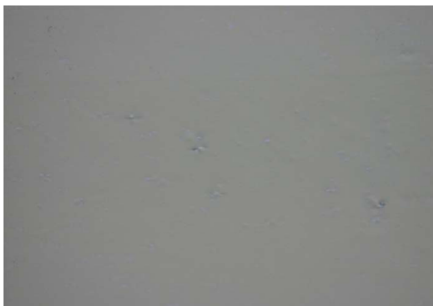
Figure 5 Air bubbles due to poor adhesion of white surface film
